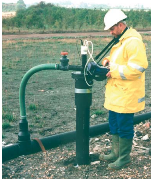
Figure 2: Landfill gas monitor and borehole
